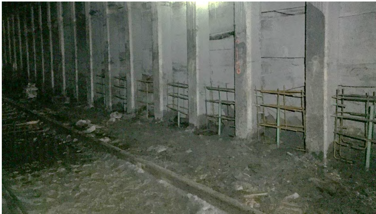
Photo: Tunnel 13, Installation of rebar cages and micropiles in preparation for concrete.
