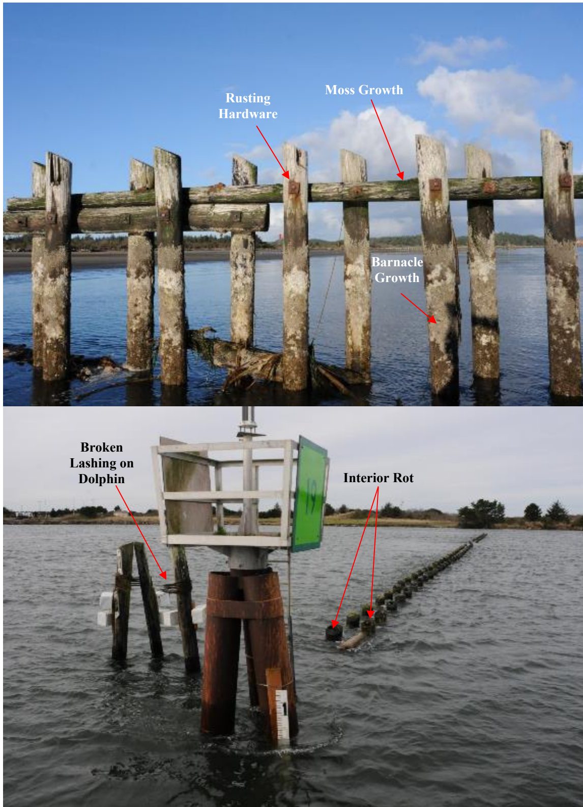
Figure 23. Pile Dike 6.8 photographs depicting the condition of the piles and hardware.
