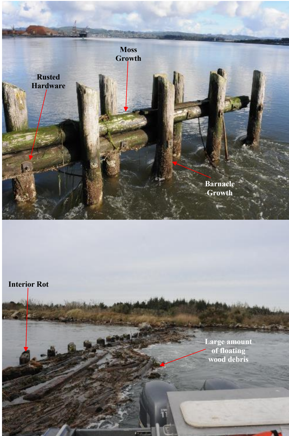
Figure 36. Pile Dike 7.3 photographs depicting the physical condition of the piles, hardware and floating debris during an ebb tide.
