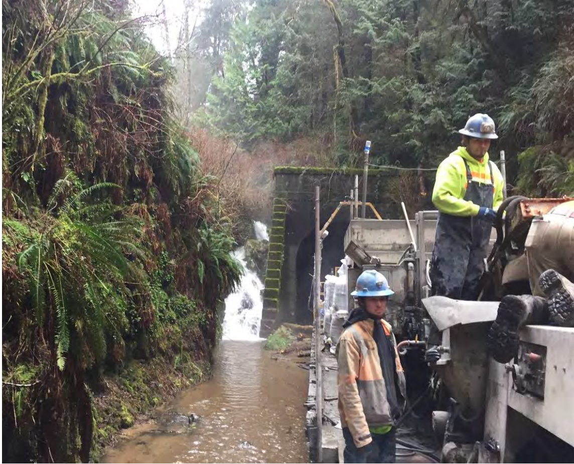
Photo: Tunnel 19, Outside the South Portal, looking north from the shotcrete work train.
