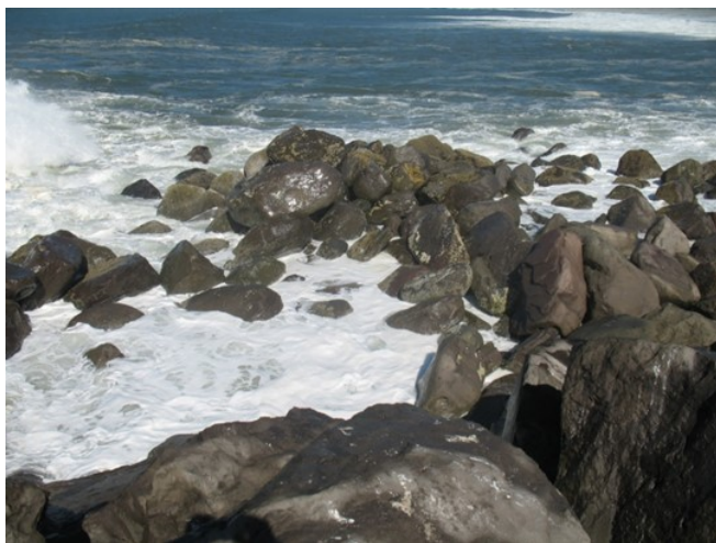
Figure 2-36 Displaced Stone Adjacent to Reach N2c, Channel Side, October 2010
