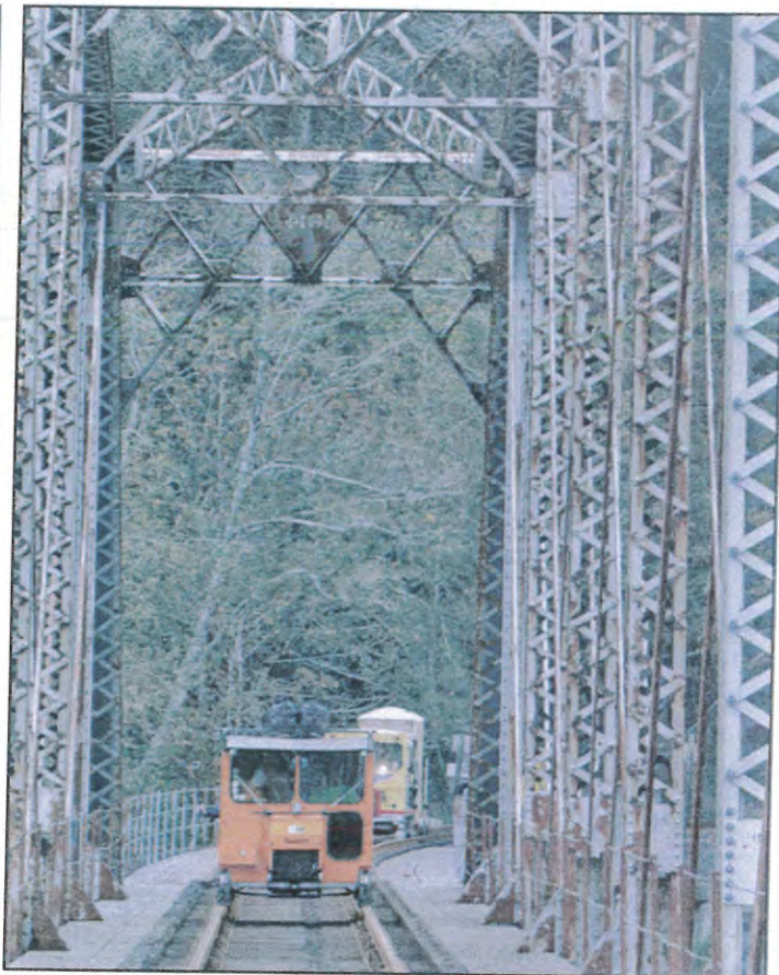
All of the CBRL through truss and swing bridges were built by the American Bridge Co. in 1914. The lack of maintenance over the years, by previous owners, is painfully obvious.
