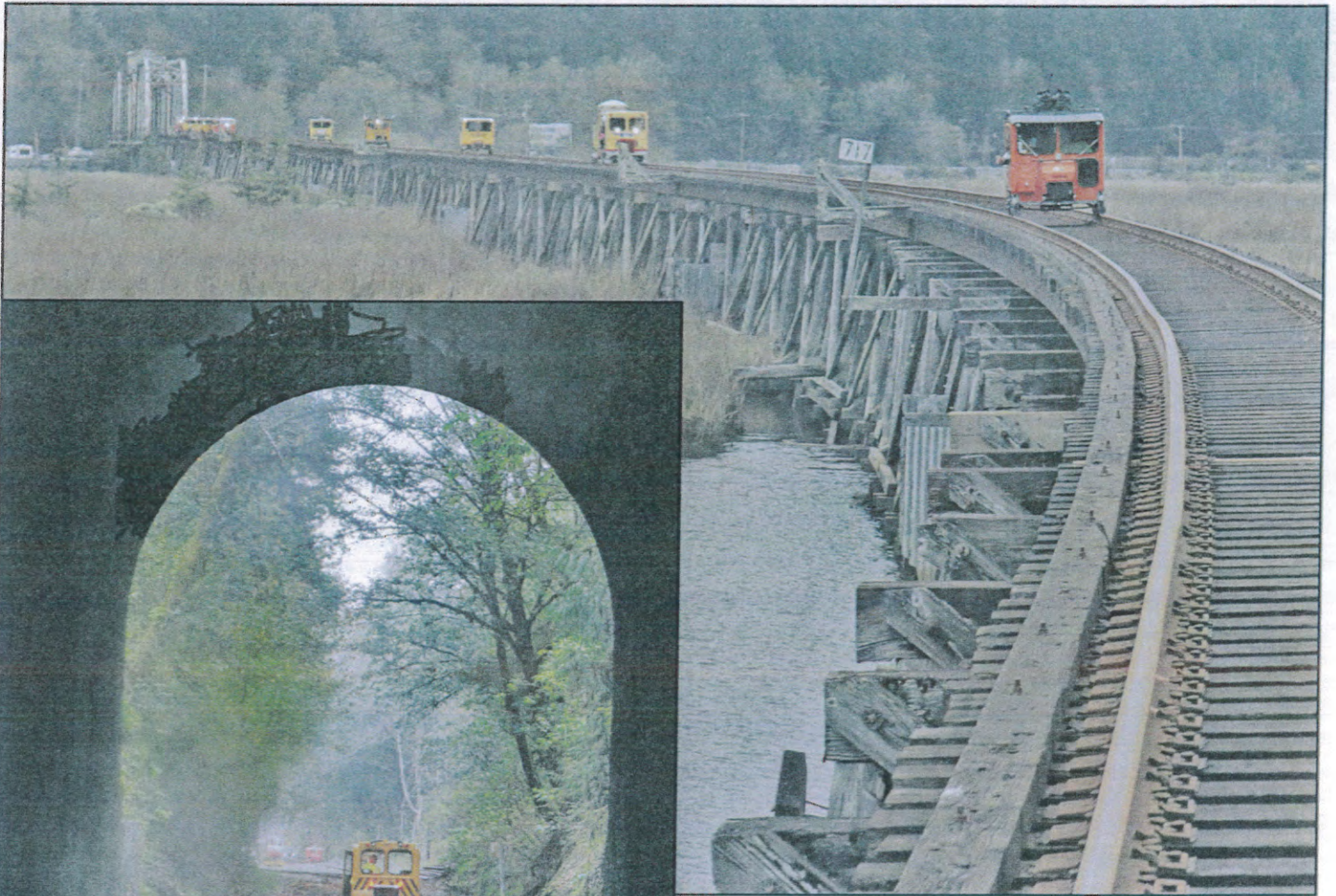
Above: At 3450 feet, the Siuslaw bridge, with a 295-foot swing span, is the longest bridge on CBRL. The swing span is no longer used.
