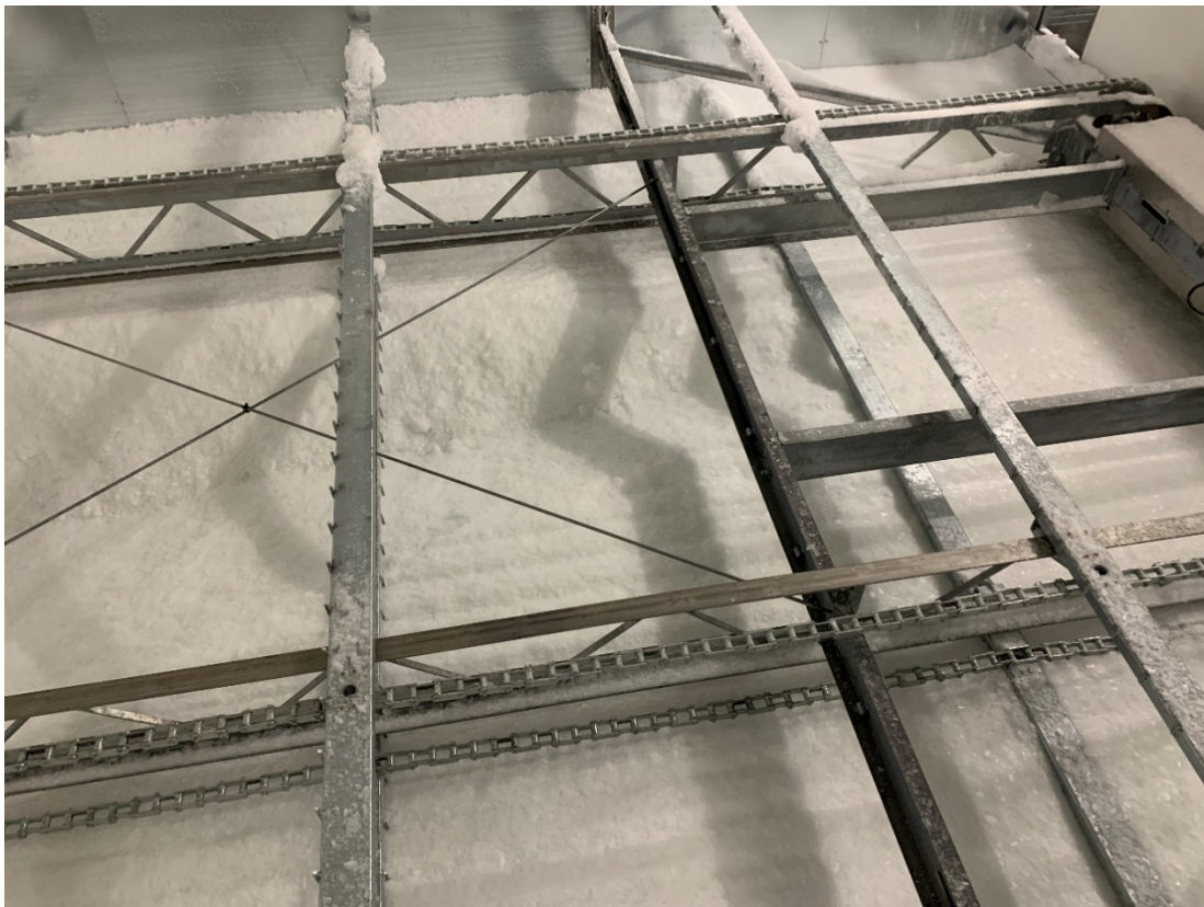
Photo: Ice rake system in the new plant, September 2020.
