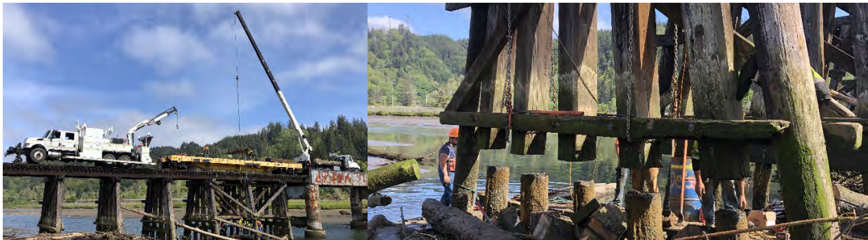
(Contractor affecting same repair to another bridge some years earlier. Old sill removed and was replaced with a new one.)
