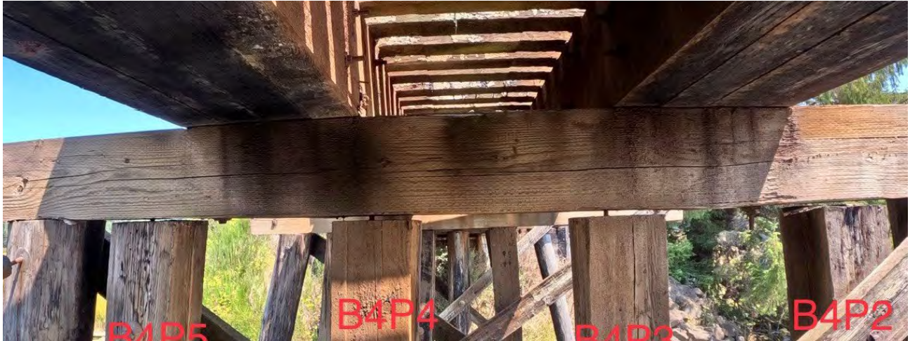
(Gaps appearing due to posts settling because of sill failure MP 739.43. This allows bridge to “flex” under the weight of the trains causes crushing and eventual failure of the caps and posts.)
