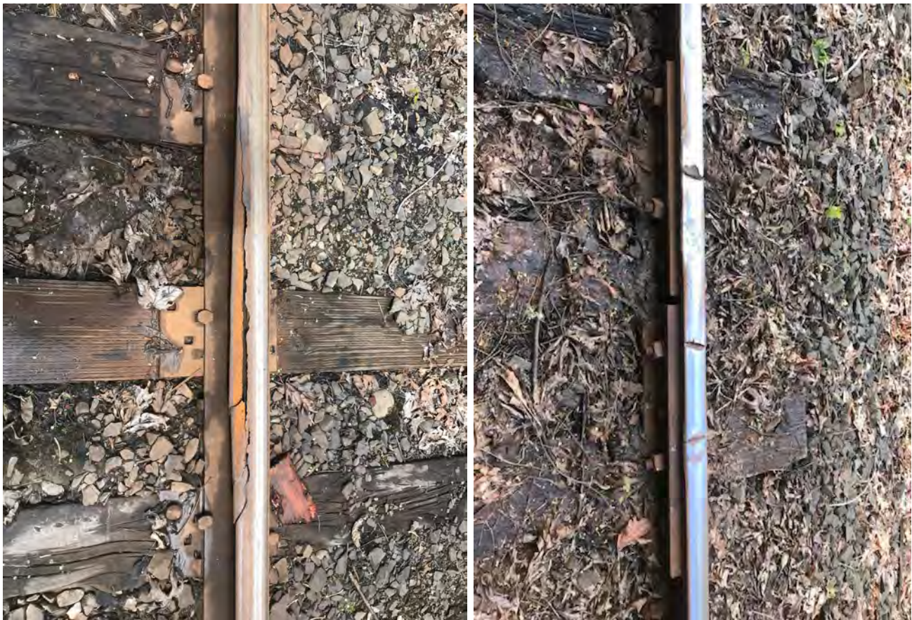
Examples of broken rail at 2 locations
